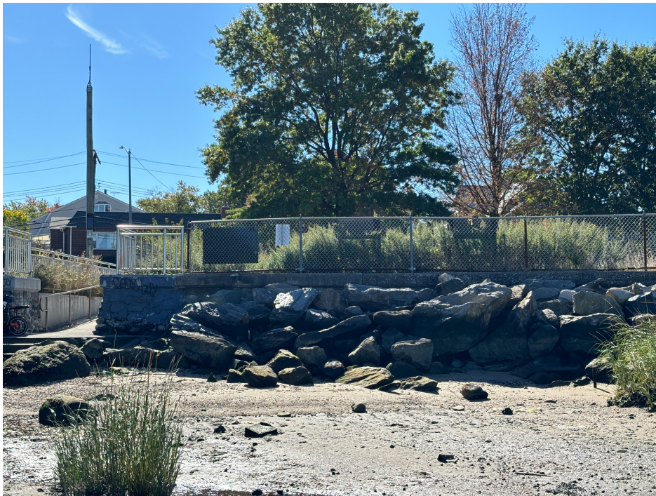
Figure 23. The seawall at Hermon A. MacNeil Park from the perspective of the East River. The ramped entrance bisecting the wall is at the far-left of the image.
