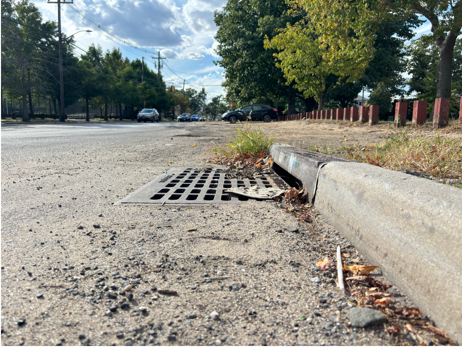
Figure 20. The catch basin on 147th Ave by Brookville Park.
