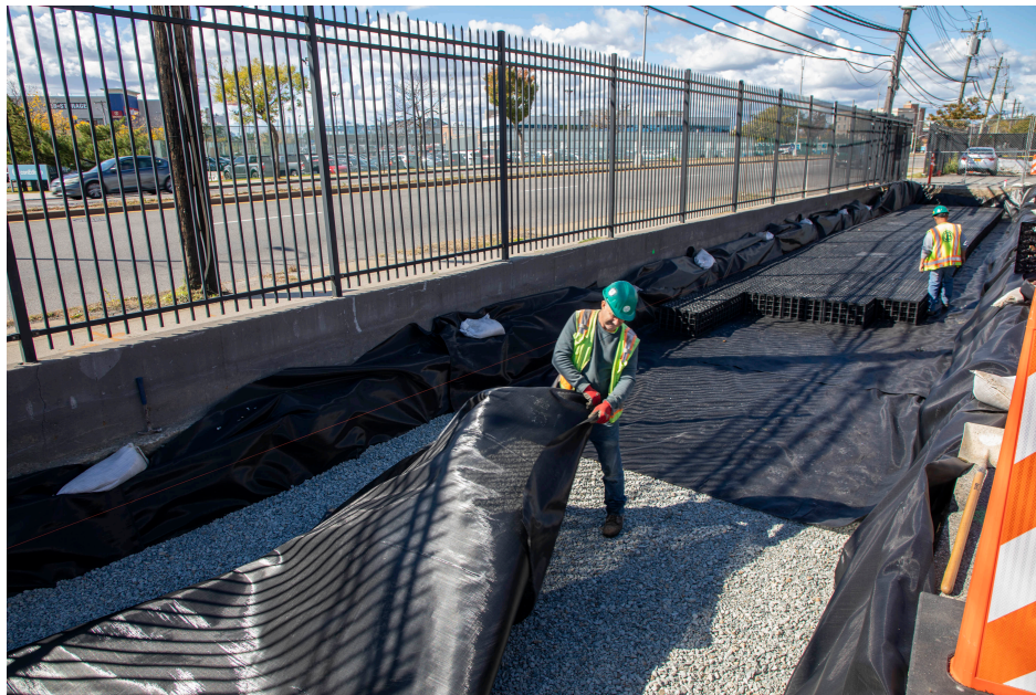
Figure 28. Workers installing porous pavement at a parking lot in College Point, Queens.
